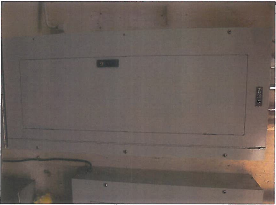
EXISTING PANEL "PP"
