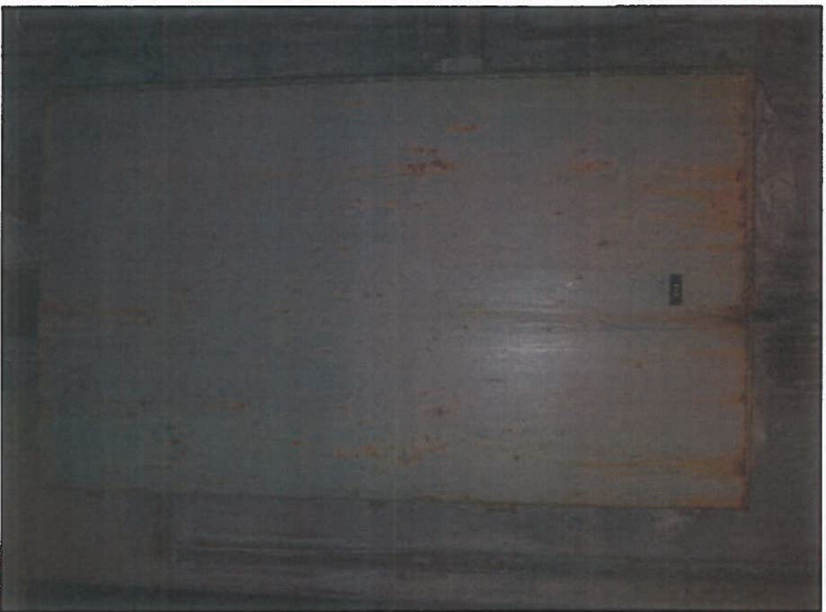
EXISTING PANEL "F1"
