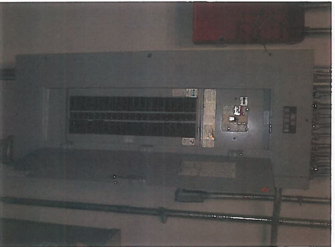
EXISTING PANEL "EKAP"
