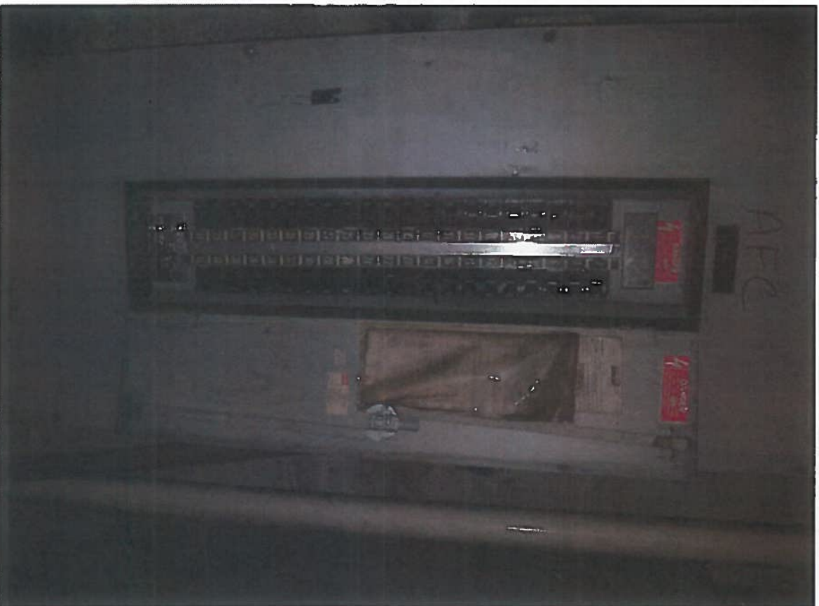
EXISTING PANEL "F"
