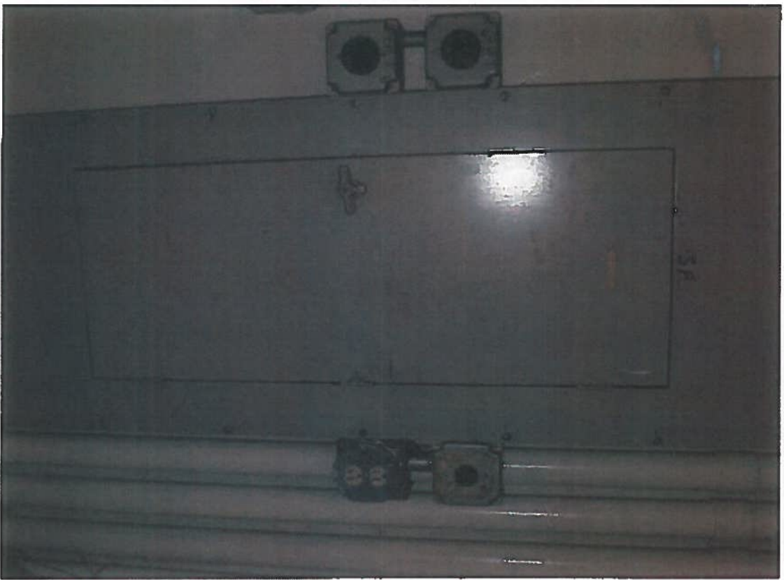
EXISTING PANEL "SF"
