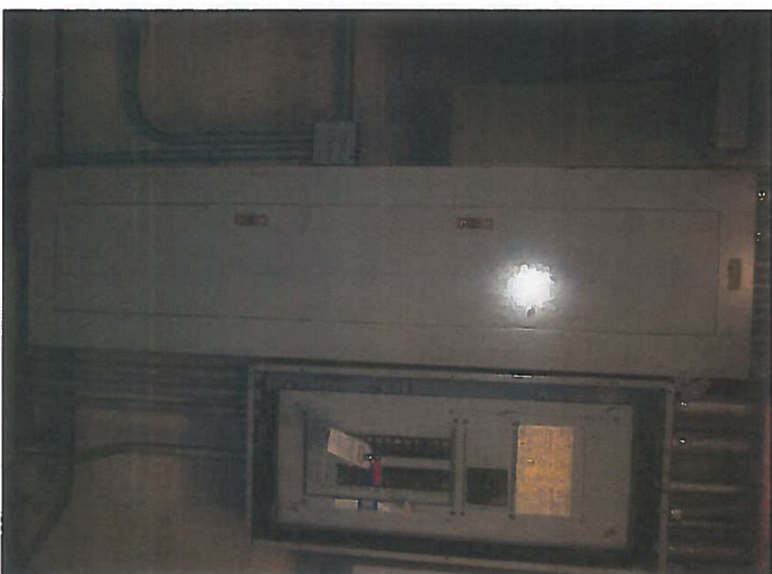
EXISTING PANEL "AFC"
