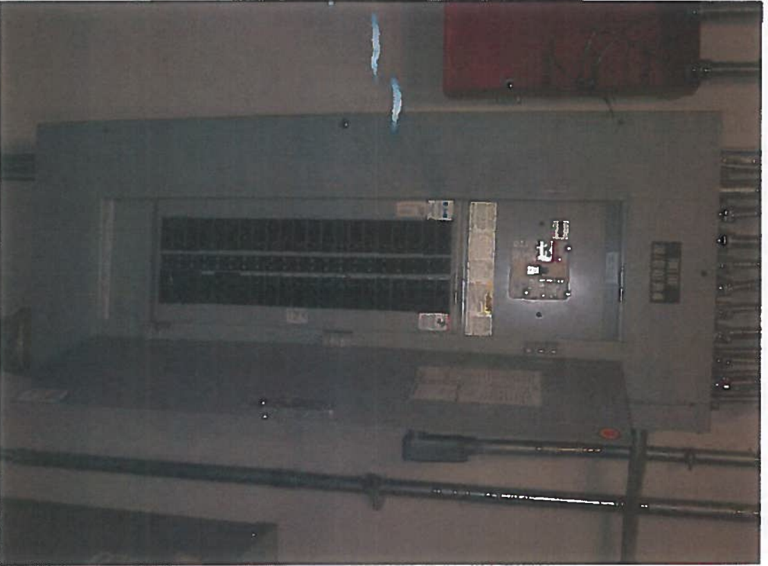
EXISTING PANEL "EKAP"
