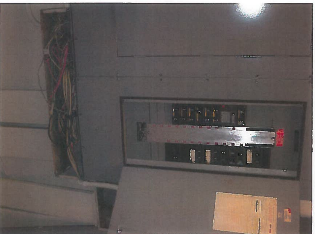
EXISTING PANEL "NMF-2"
