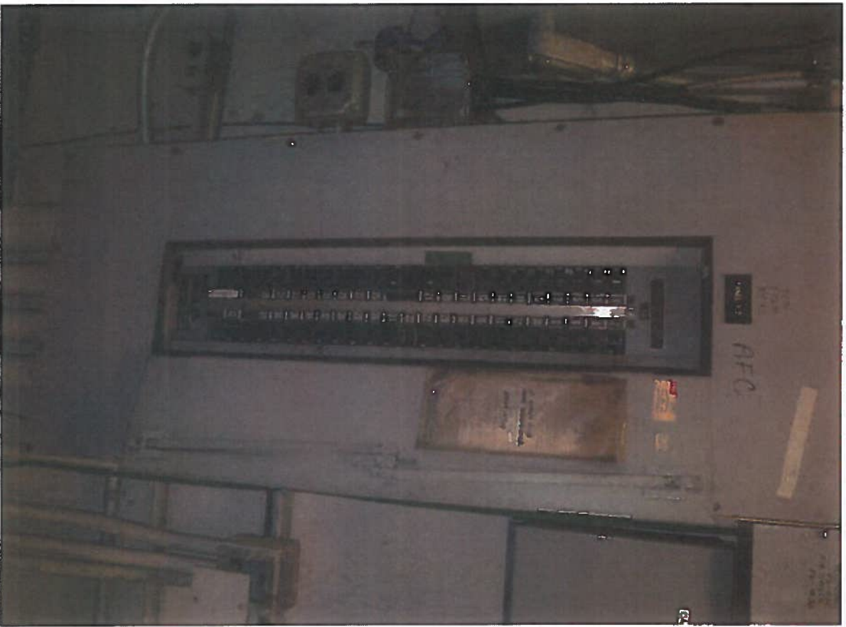
EXISTING PANEL "F2"
