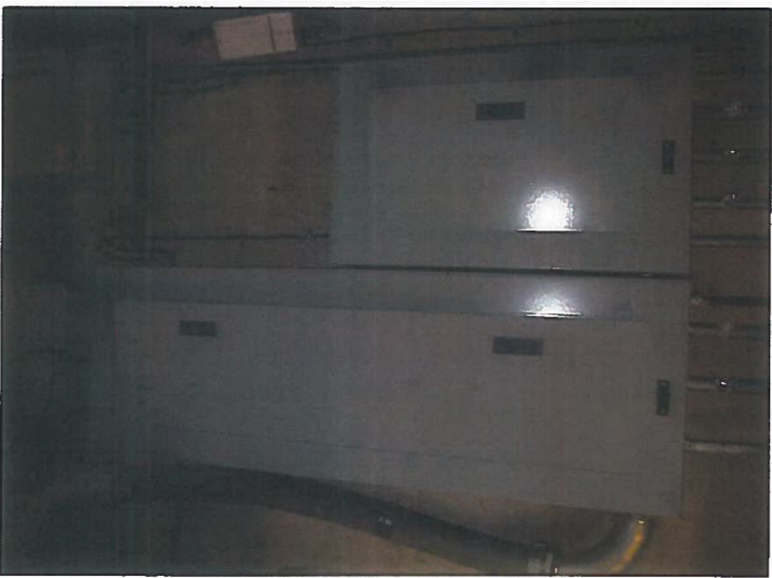
EXISTING PANEL "F1"
