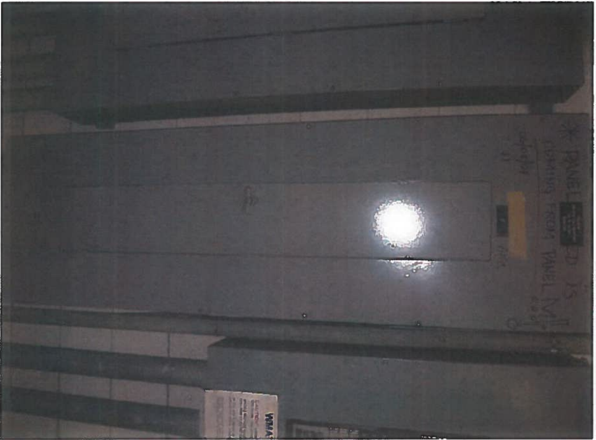
EXISTING PANEL "F"
