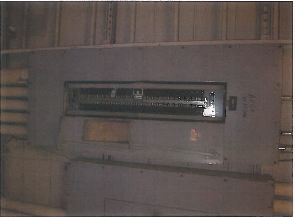
EXISTING PANEL "F1"
