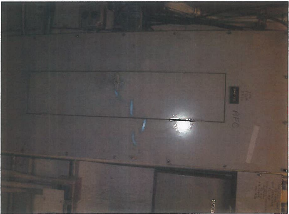
EXISTING PANEL "F2"
