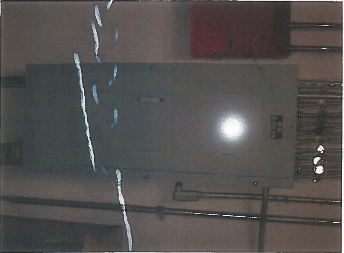
EXISTING PANEL "EKAP"
