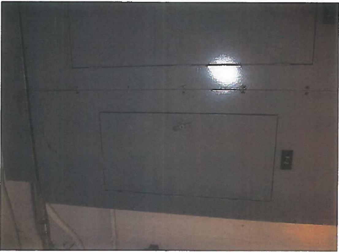
EXISTING PANEL "F-2"
