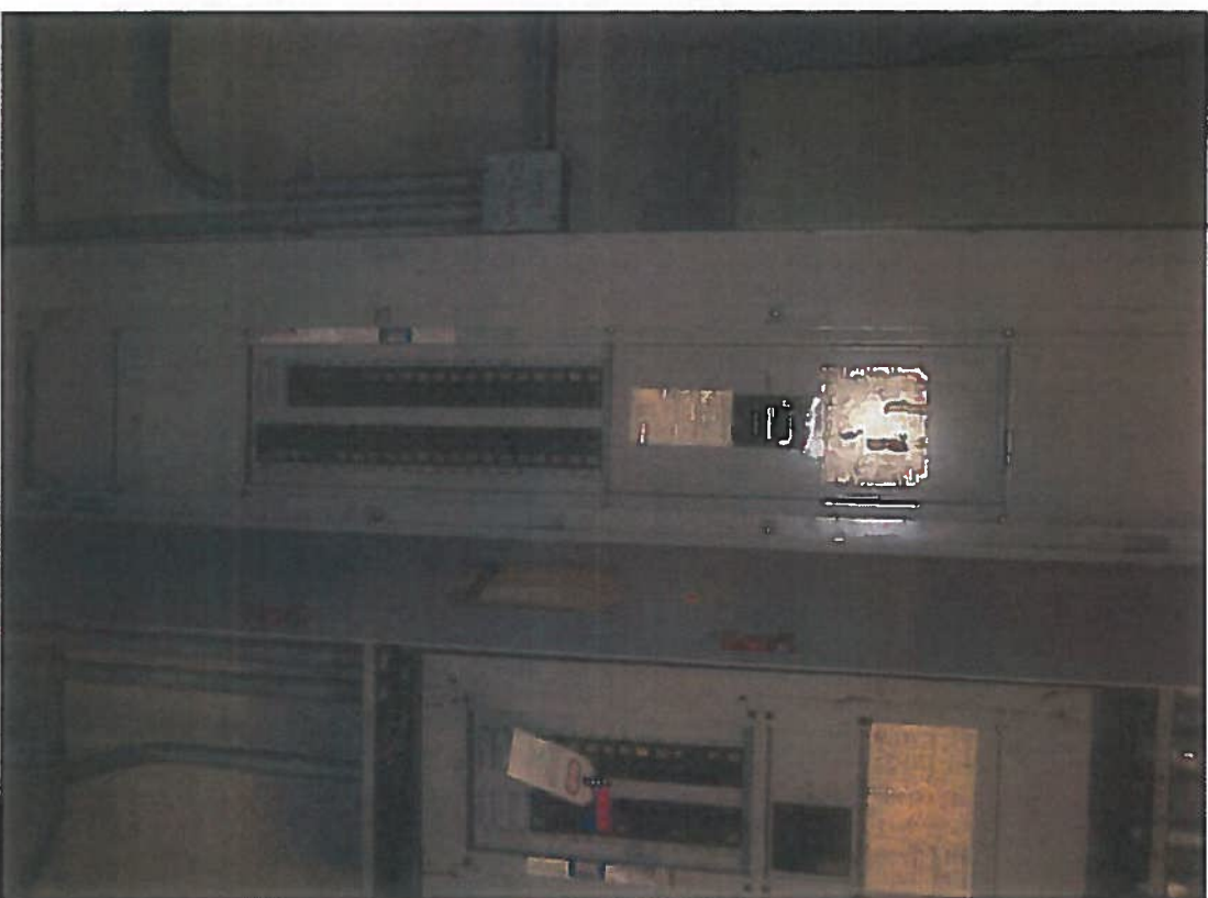
EXISTING PANEL "AFC"
