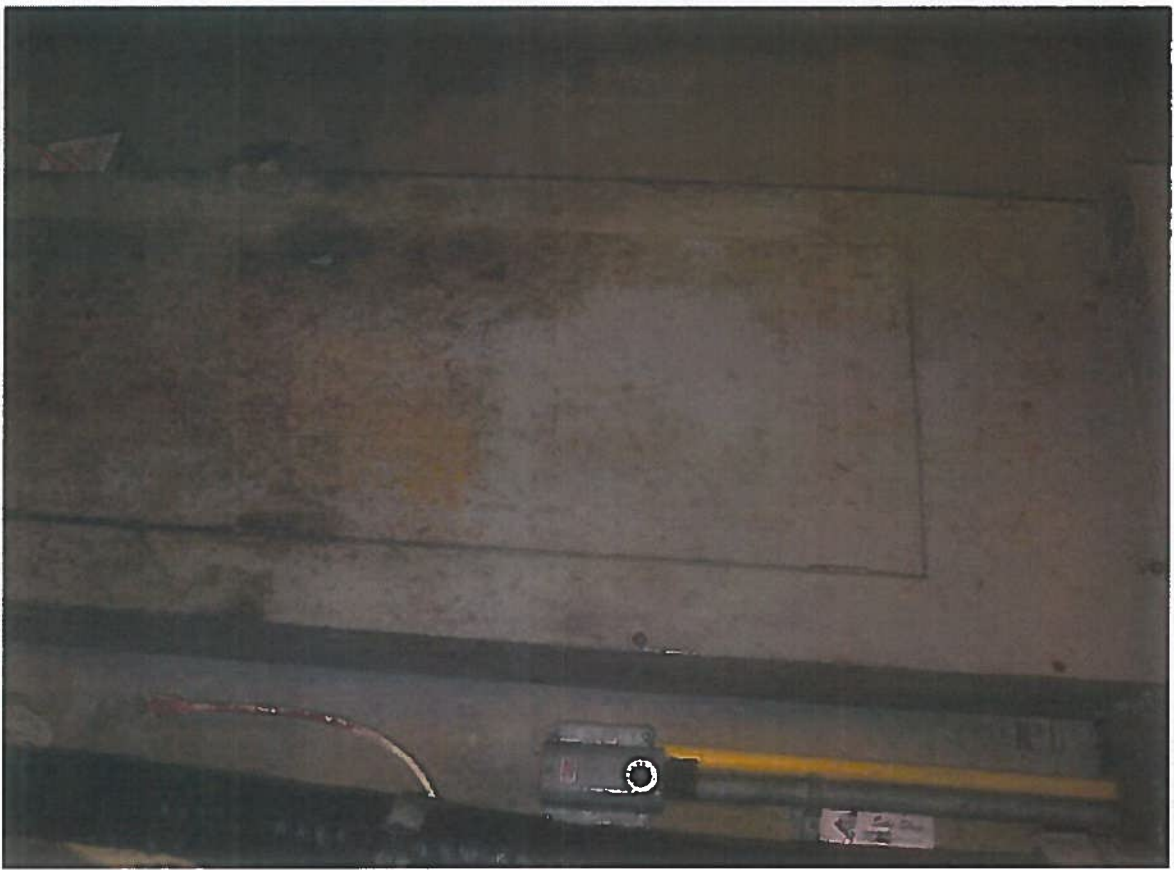
EXISTING PANEL "SF"
