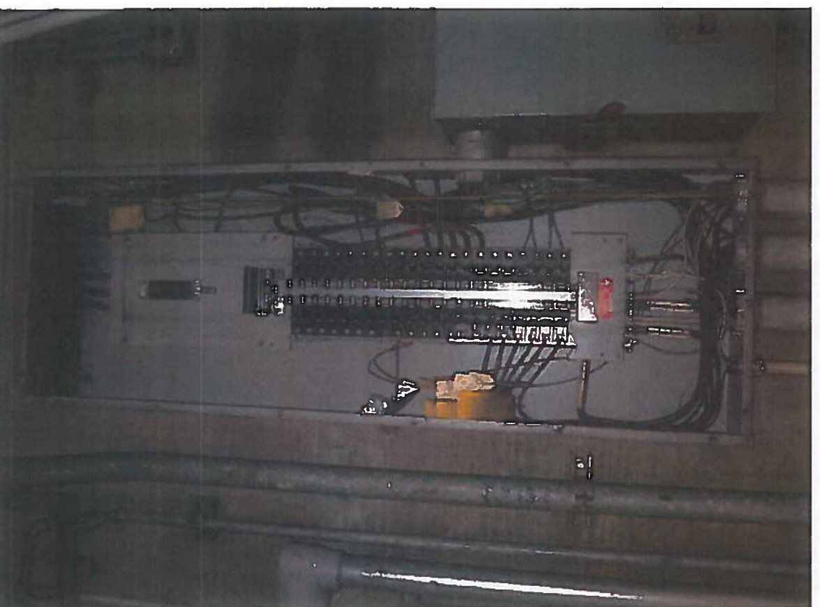
EXISTING PANEL "F"
