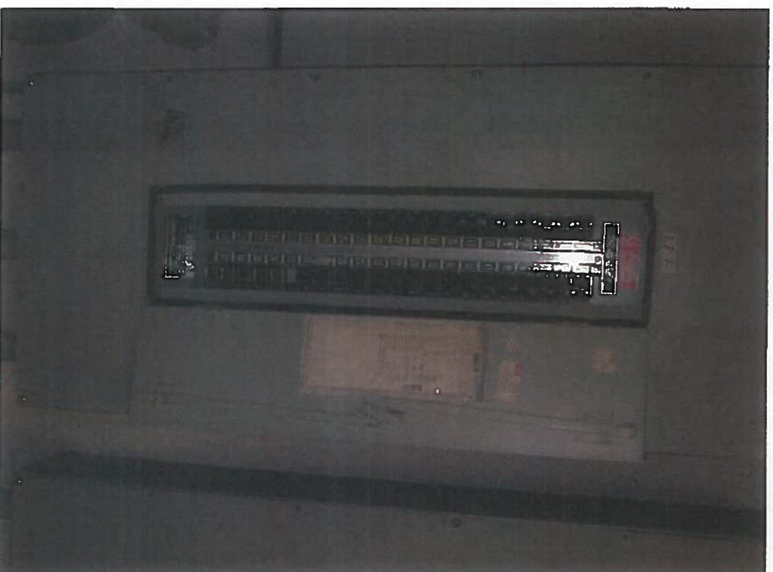
EXISTING PANEL "LP-F"
