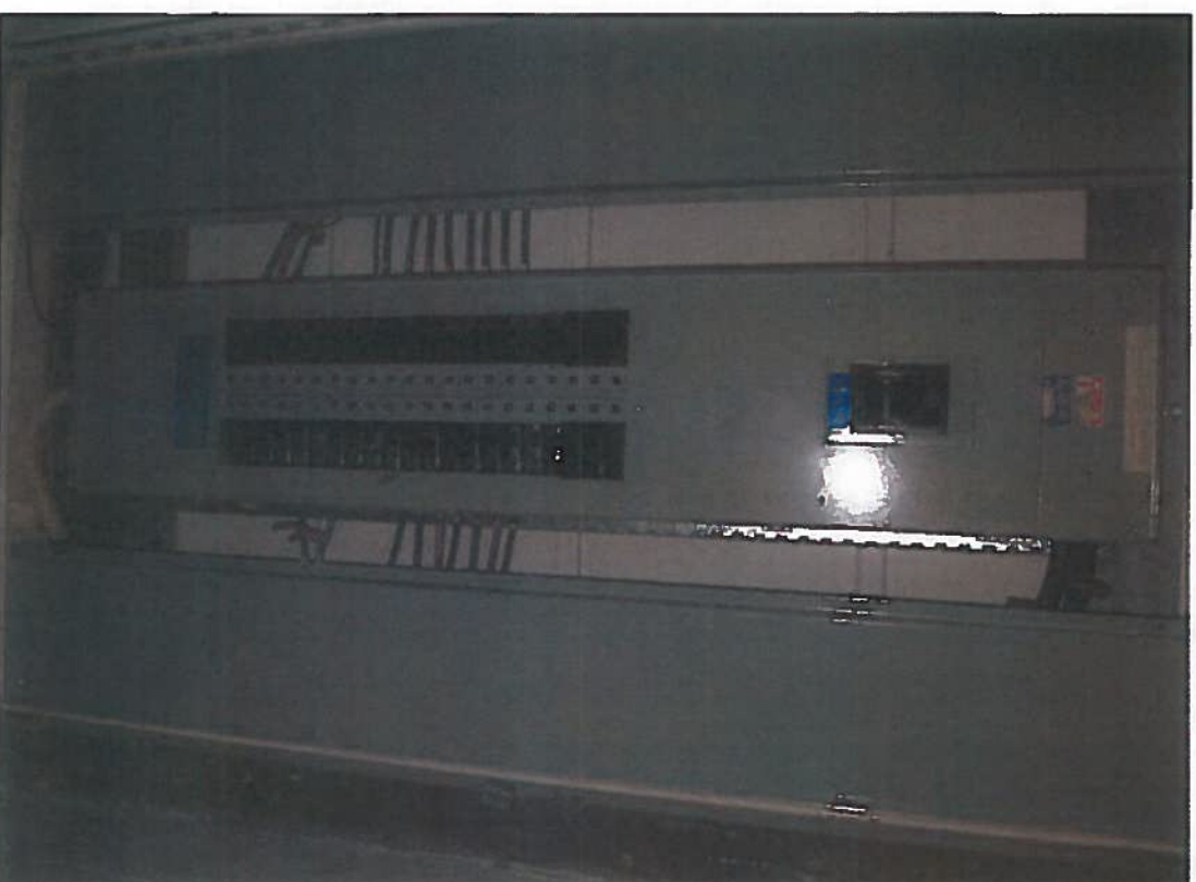
EXISTING PANEL "F1"
