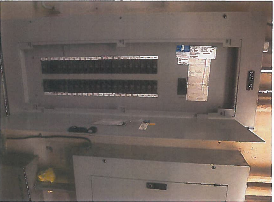
EXISTING PANEL "PP"
