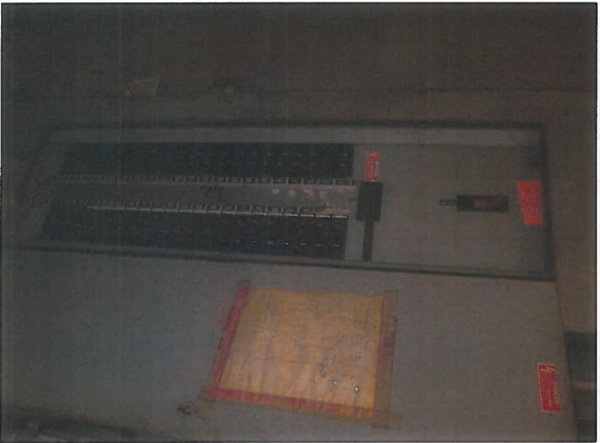
EXISTING PANEL "SF"
