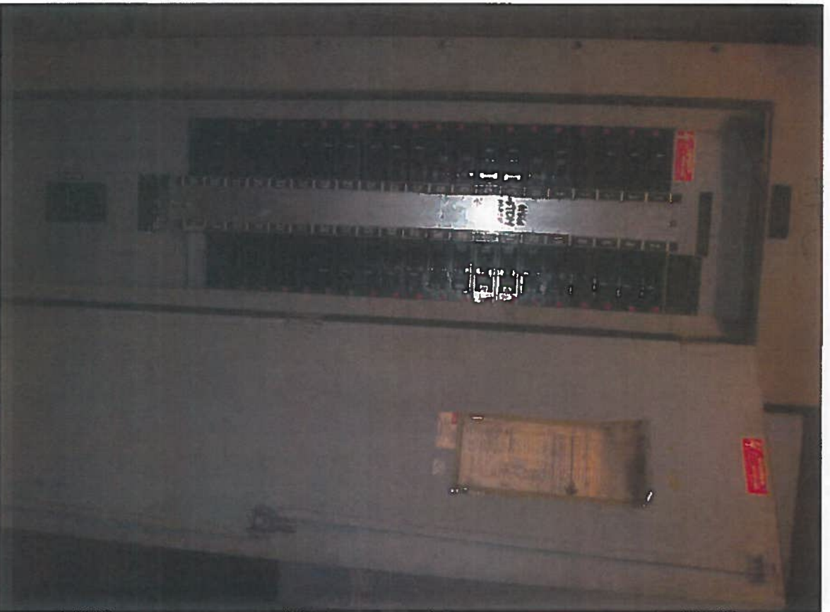
EXISTING PANEL "MNCC"
