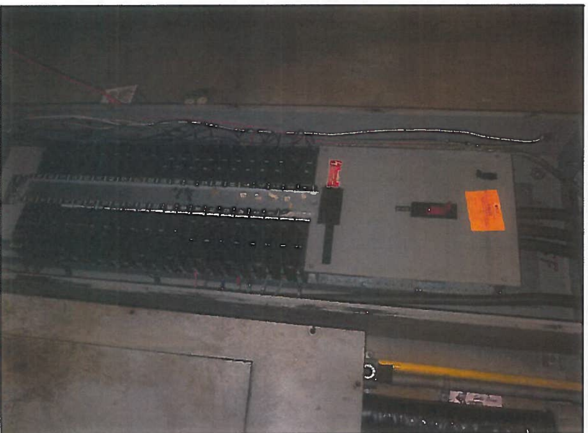
EXISTING PANEL "SF"
