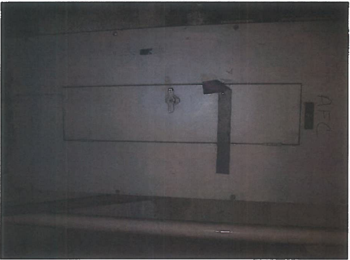
EXISTING PANEL "F"
