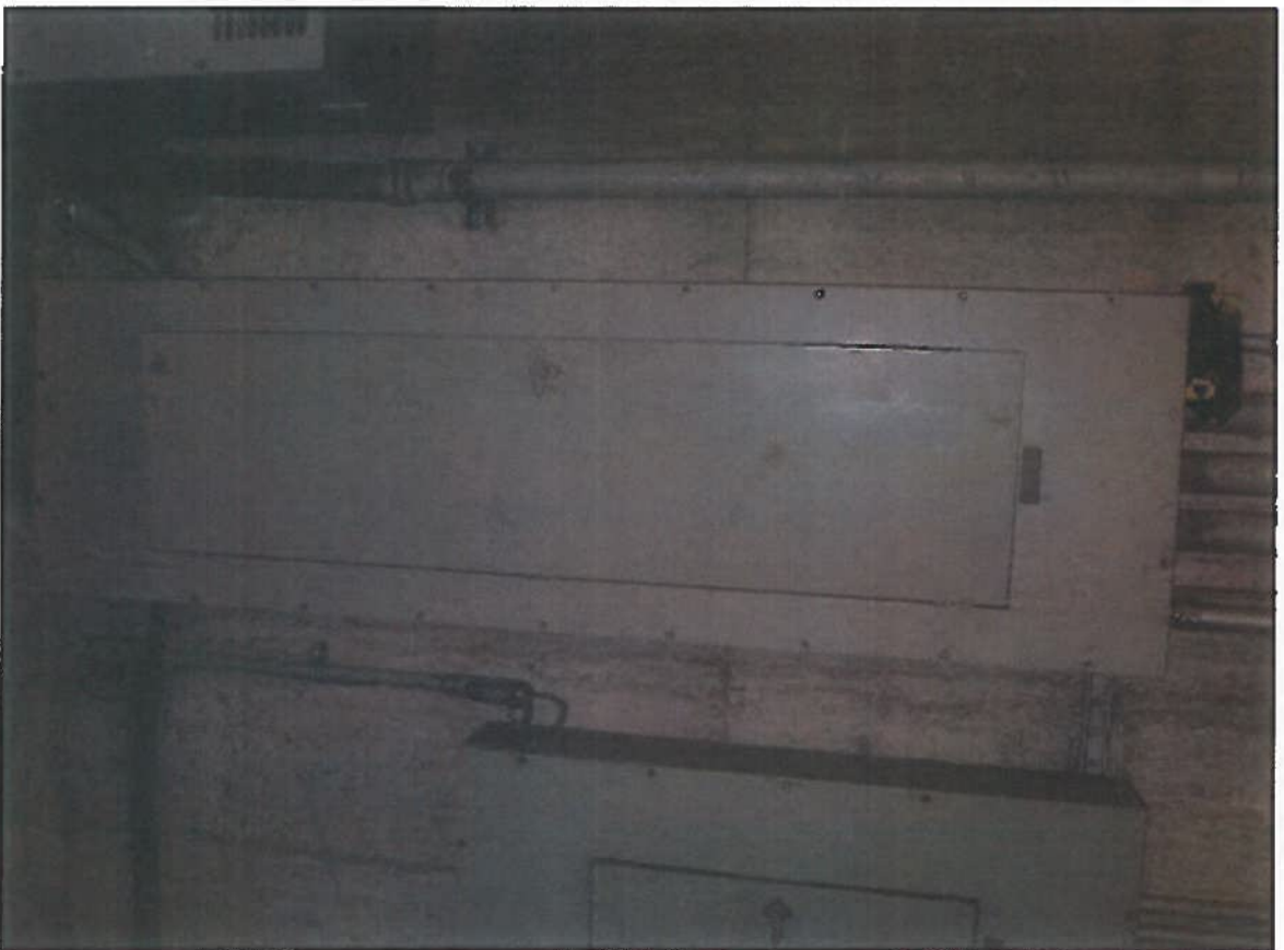
EXISTING PANEL "MSAA"
