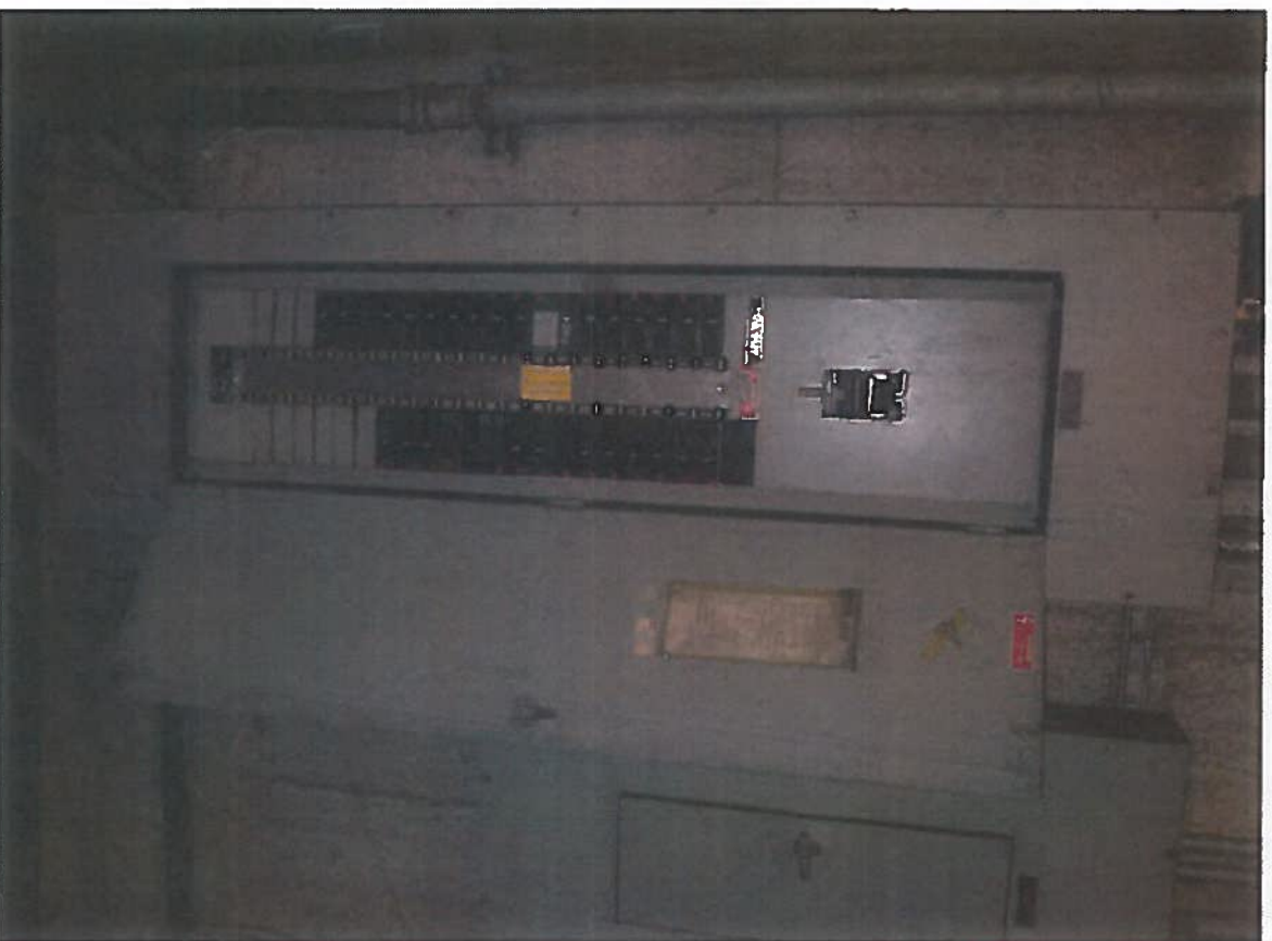
EXISTING PANEL "MSAA"
