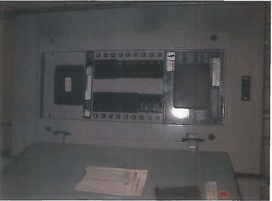
EXISTING PANEL "F1"
