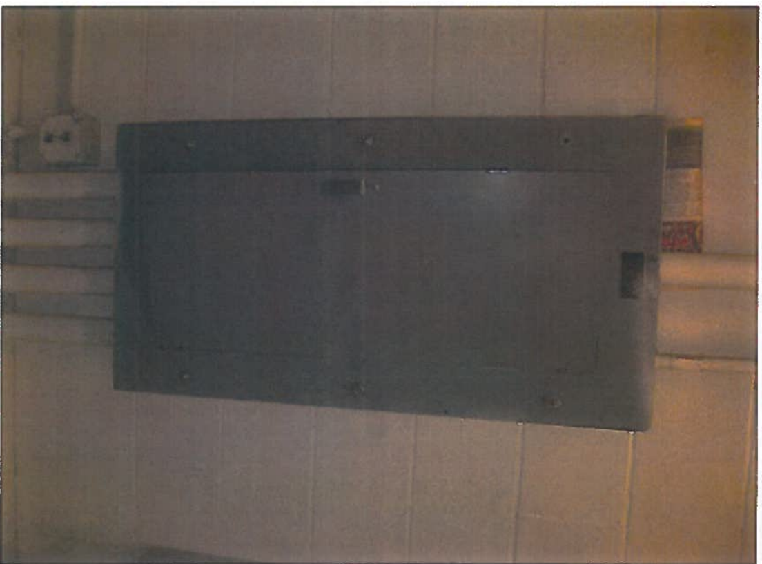
EXISTING PANEL "LP-F"
