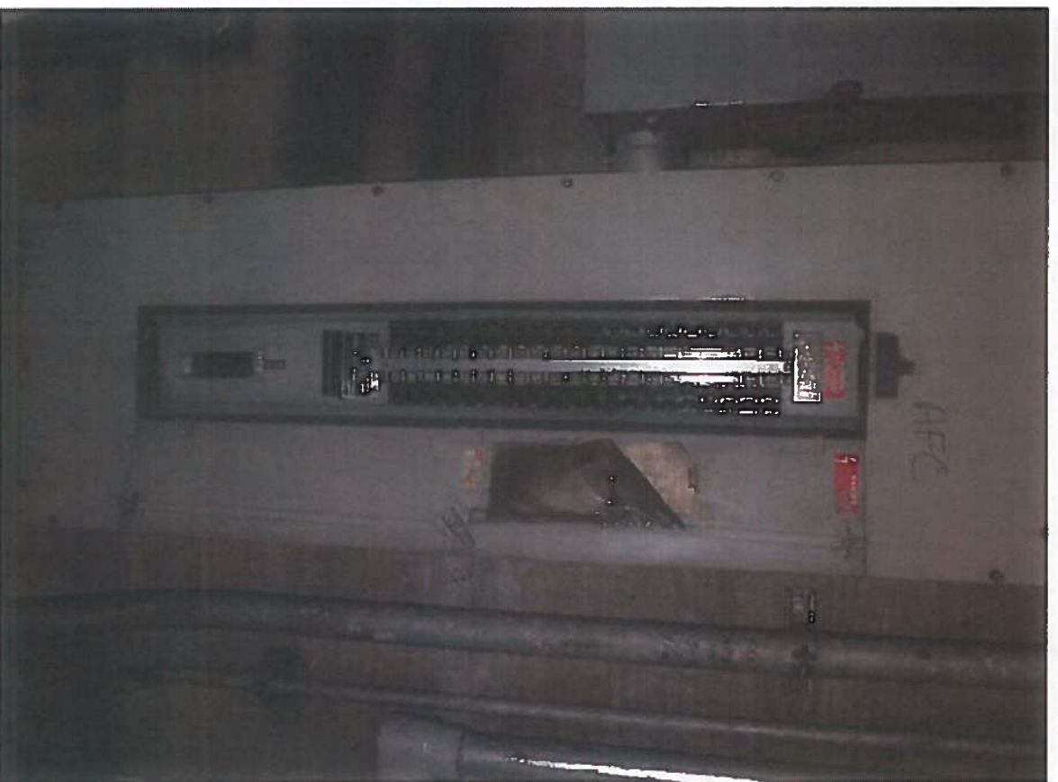
EXISTING PANEL "F"
