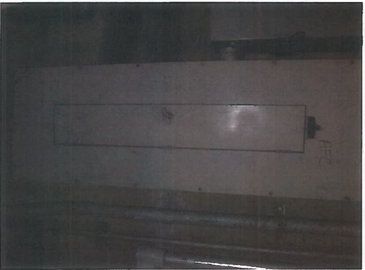
EXISTING PANEL "F"
