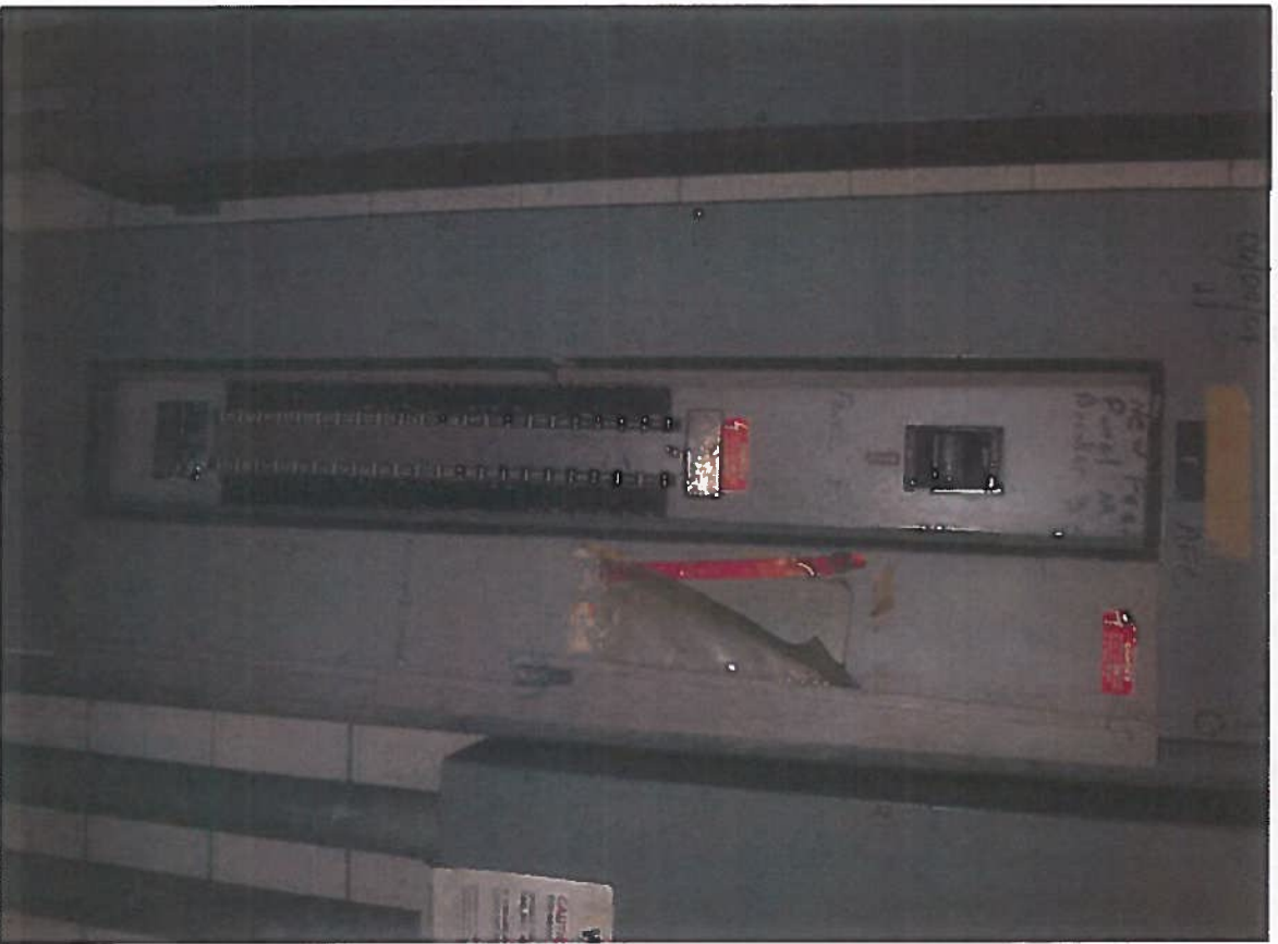
EXISTING PANEL "F"
